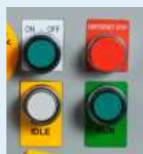
Control panel labelling
