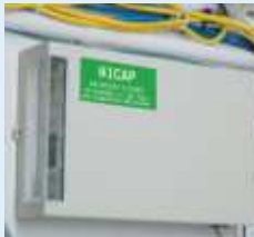
Control panel labelling
