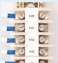
Terminal block marking
