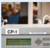
Control panel and electrical panel labels
